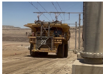
Hot commissioning on Trolley Line#05 with Haul Truck#22
