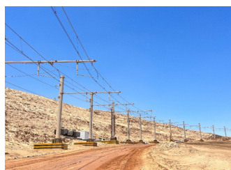
Trolley Line#04 in Z2S4
