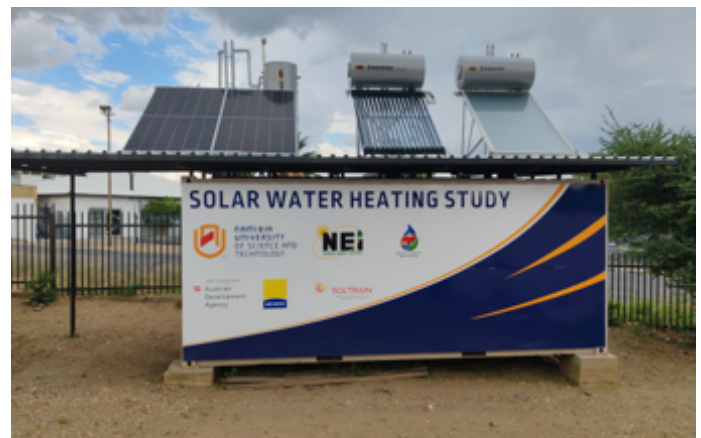
A Real-World Comparative Study of Different Solar Water Heating Systems under the SOLTRAIN Project.
